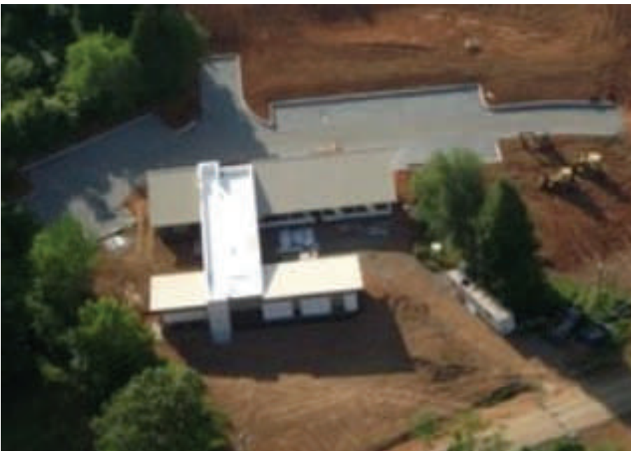
Soaring to Completion – a bird's eye view of our new Tellico Village Public Library, courtesy of Warren Parthen taken from his powered parachute. [Submitted by Kathy Economy]
